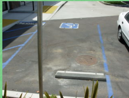
Manhole cover on surge tank under parking space – photo from ReWater, Inc.
