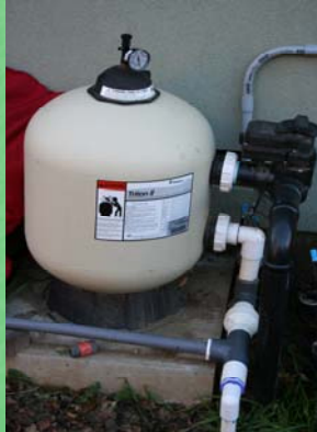
Sand filter from ReWater
