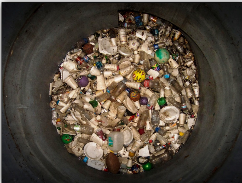
Photo 3: Lighter Materials in a Hydrodynamic Separator within the San José Storm Drainage System
