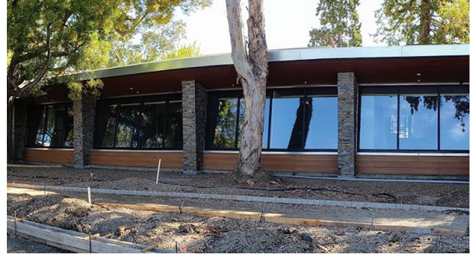
With our growing City, continuing to create and expand spaces for people to come together, celebrate, and share ideas has never been more important. The Mountain View Community Center expansion is well under way and is expected to reopen to the public in the first half of 2019.
