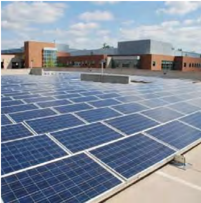
Rooftop solar panels in North Bayshore.
