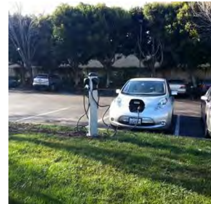
Typical electric vehicle charging station.
