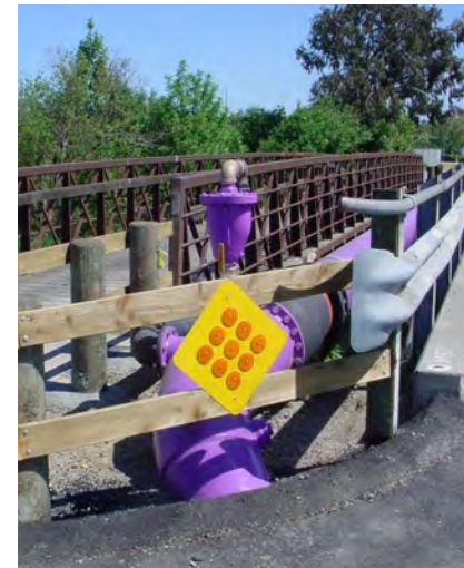
North Bayshore is served by a recycled water system.
