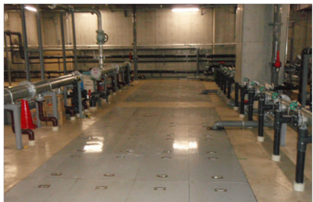
Figure 2 View of the MBR system installed (Photo credit: Drico. Ltd.)
